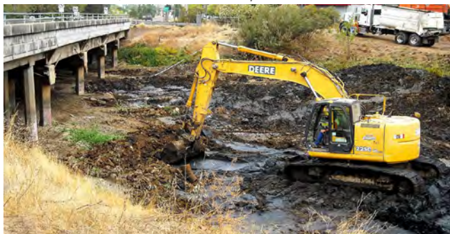
The Department of Public Works Water Resources team preventative maintenance and construction.
